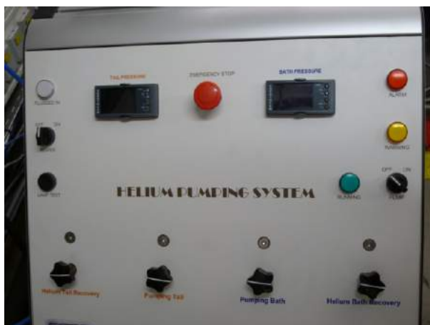
FIGURE 8.12.5 – Banc de pompage
